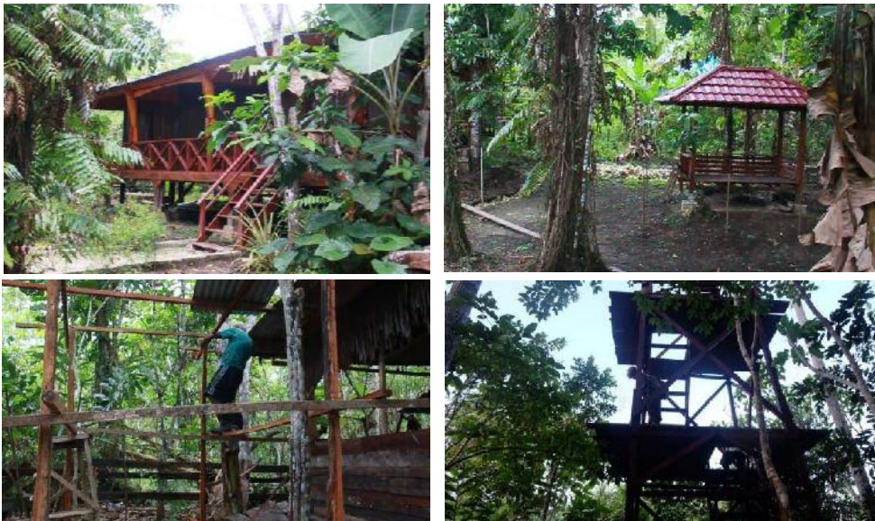
Figure 81 A cottage in Isyo Hill (top left); gazebo (top right); process to build public kitchen (bottom left); tower for birdwatching (bottom right)
